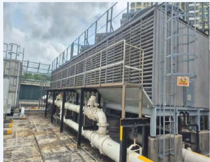
Figure 2: Provision of catwalk for safe, efficient, and effective cleaning of cooling tower fill media
